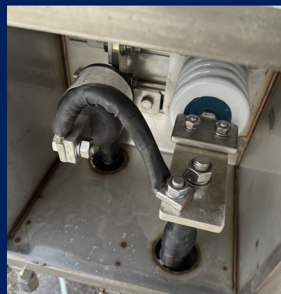
Sheath voltage limiters (correctly in service position)
