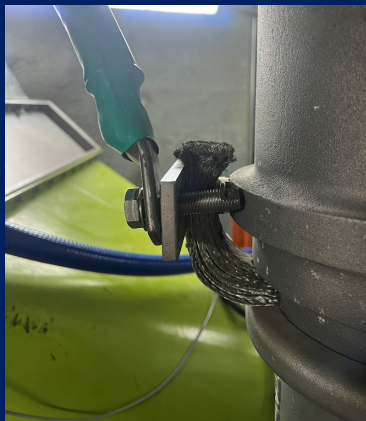
Bolted earth (shown test fitting new bolt for padlocks)
