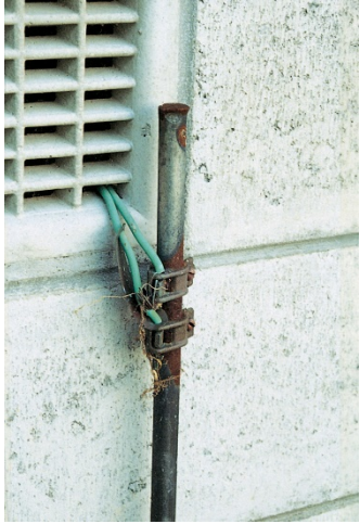
Corroded, Loose or Broken Earth Wires
